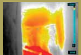
Heat Seeker PLUS in Low Sense Mode: Notice wall and ceiling separation
