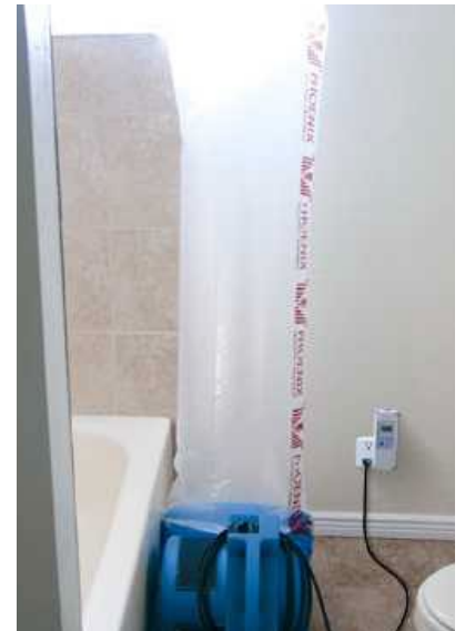
Air mover with ducting connected to Exhaust Controller
